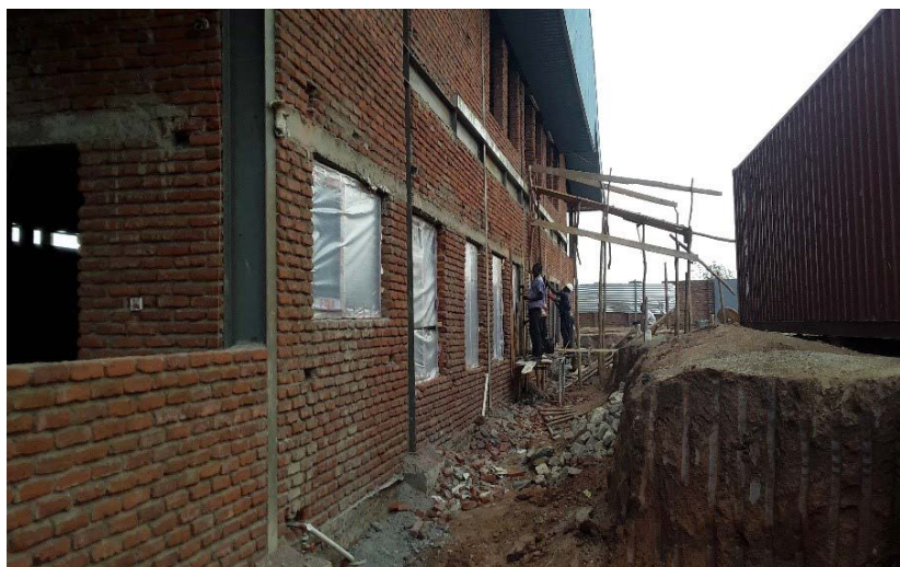
AISL Laboratory under construction in Kanengo Lilongwe. The expected completion date is January 2018 and ready for use in March 2018.
